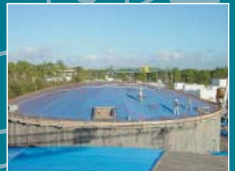
LLDPE T-GRIP™ lined Digester Dome, U.S.A.
