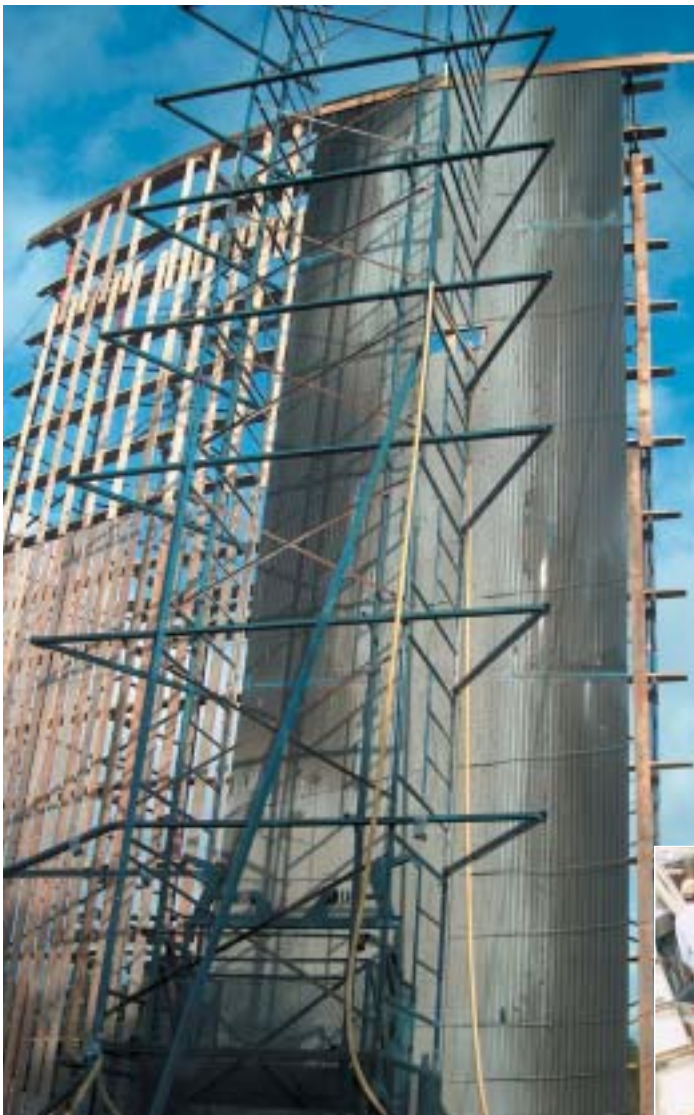
Innovative digester tank construction in U.S.A. with black T-GRIP™ polyethylene lining. (In U.S.A. also under the trade name Corr-Tite)
